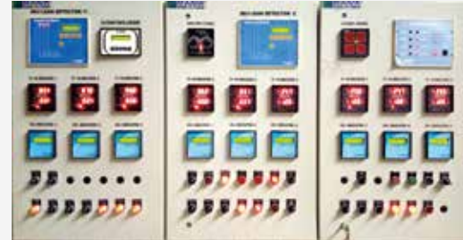
Cold Room Automation Panel
